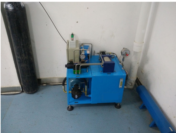
Fig. 3 Device diagram of medium and low pressure pipeline of gas booster pipeline
