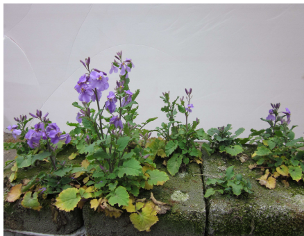
Fig. 1 O. violaceus growing on the green concrete
