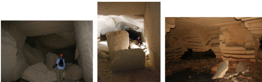
Fig. 3 Instability in calcarenite underground quarries: left : extensive failures at Altamura; center : falls from ceiling and walls in a quarry at Cutrofiano; right : wall failures in a quarry at Gallipoli
