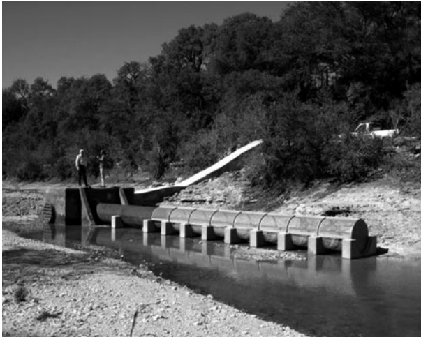
Fig. 4 Upstream view of the vault and screen constructed above the entrance to Antioch Cave. Length of intake screen is 10 m
